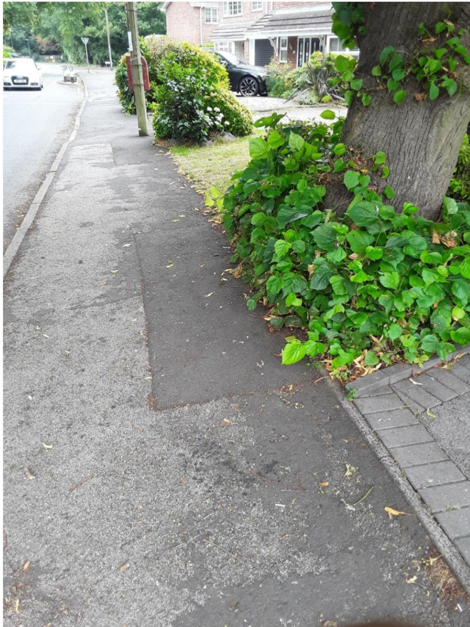
Image 3 – Showing previous rectification works to the tarmac
