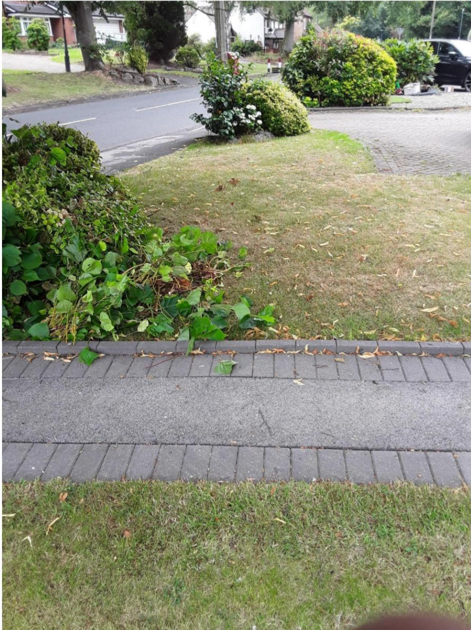
Image 2 – Showing the slight distortion on the pathway
