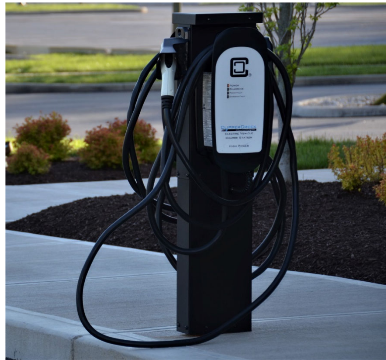
Electric vehicle charging point
