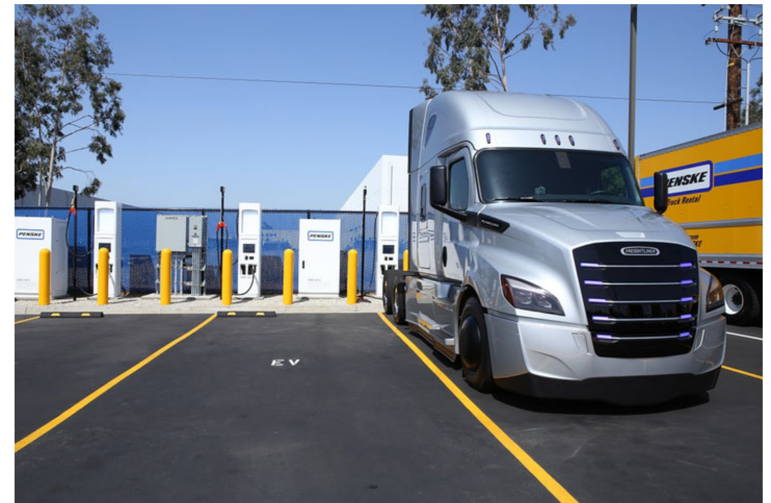
Electric lorry charging points
