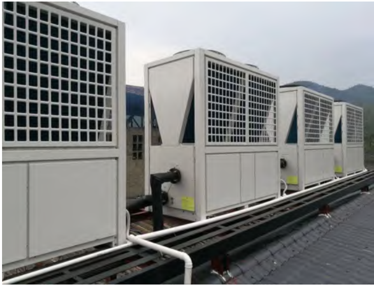
Air source heat pumps
