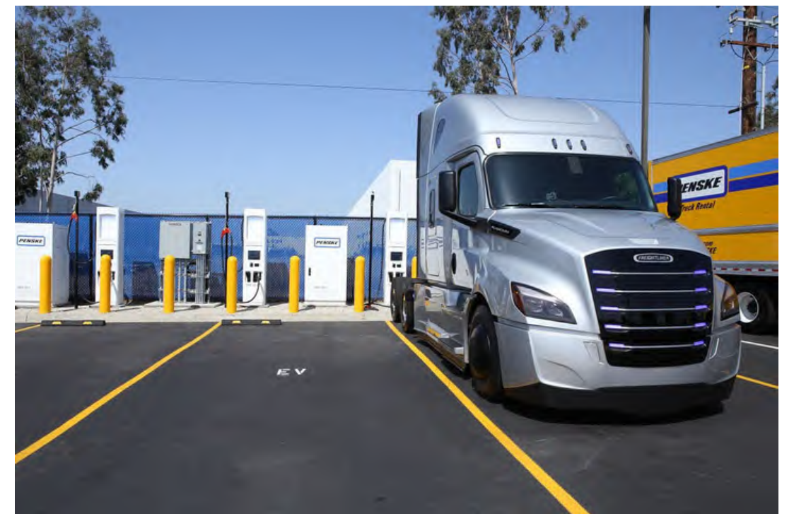
Electric lorry charging points
