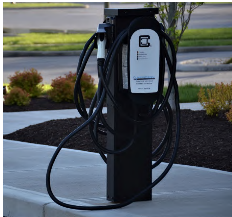
Electric vehicle charging point
