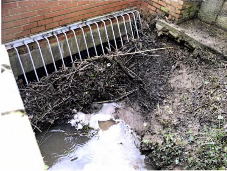
Document 3 – Photograph of Culvert Blocked with Debris
